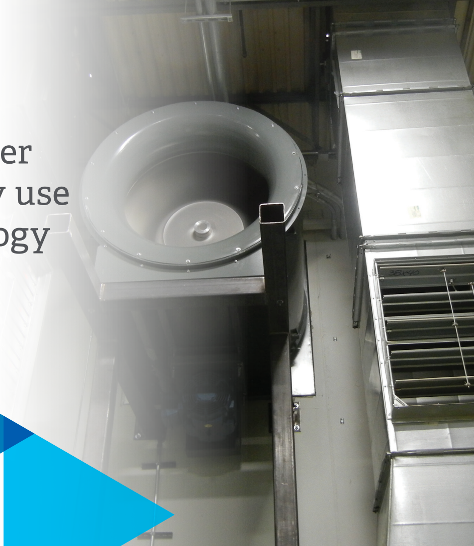
The centrifugal fan evenly distributes warm air from the compressor room.
