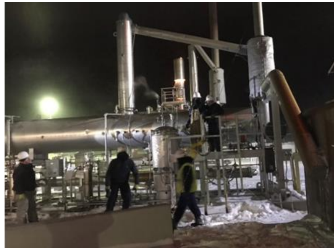
Storage reboilers are critical in maintaining gas quality during withdrawals
