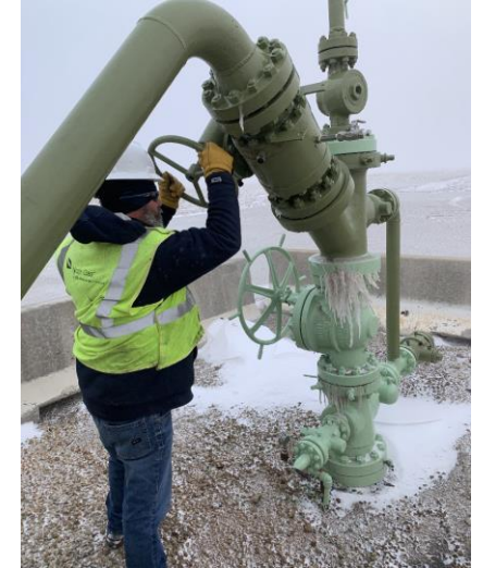
Keeping storage wells flowing
